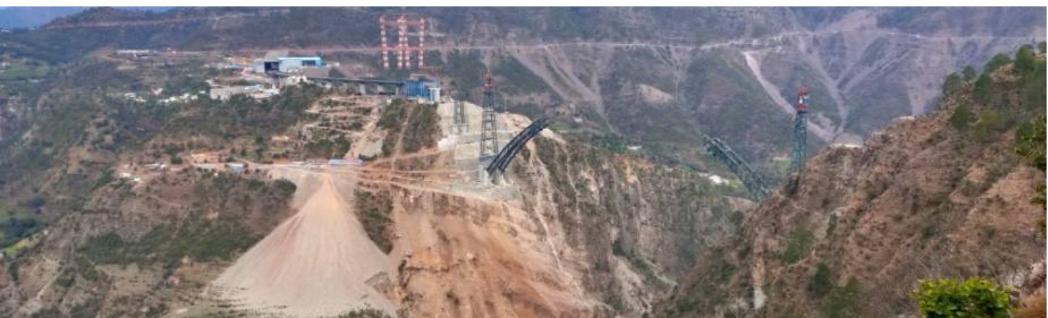
Stabilisation of the foundation and erection of the bridge were major challenges
